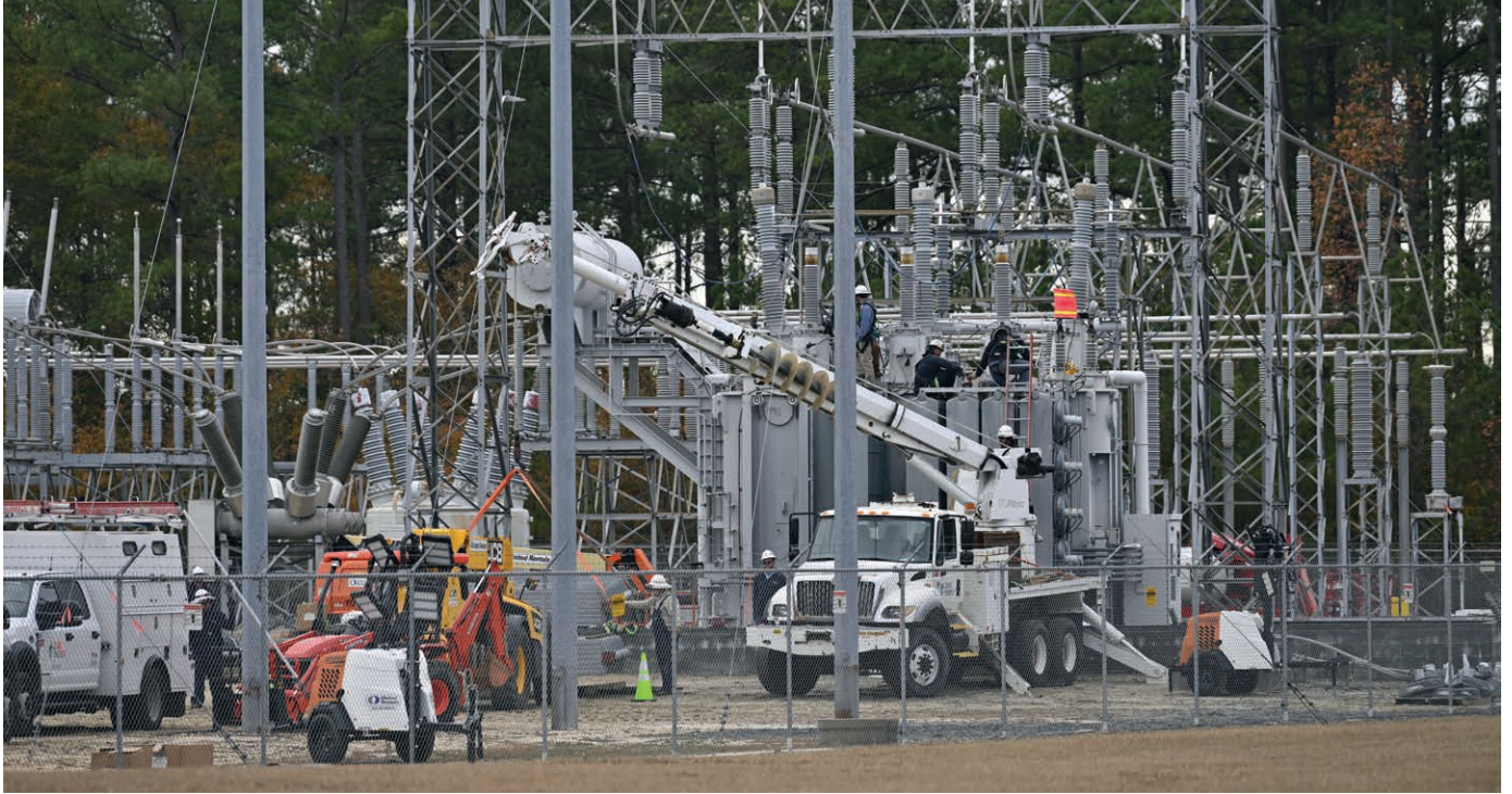
CARTHAGE, USA - DECEMBER 05: A view of the substation while work is in progress as tens of thousands are without power on Moore County after an attack at two substations by Duke Electric were shot at in Carthage NC, United States on December 05, 2022. (Photo by Peter Zay/Anadolu Agency via Getty Images)
