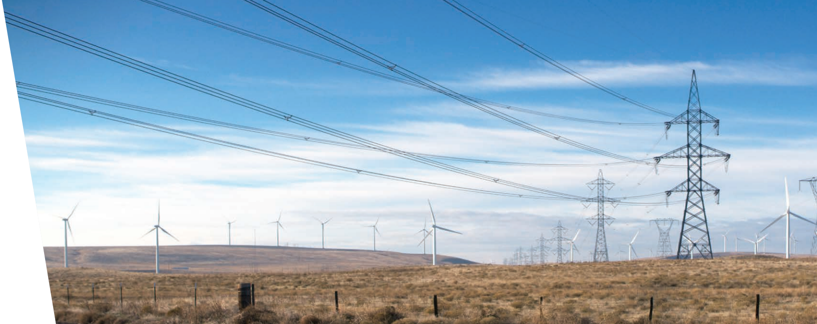
Transmission lines cross plains with wind turbines. As the United States moves to a new system of generating power, one that emphasizes the generation of renewable power and deemphasizes fossil-fueled power, we also need a new type of transmission system to move power to market. (Getty Images)
